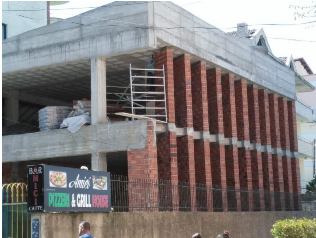
Kisha Baptiste Lajmi i Mire (Good News Baptiste Church) Construction in Progress
